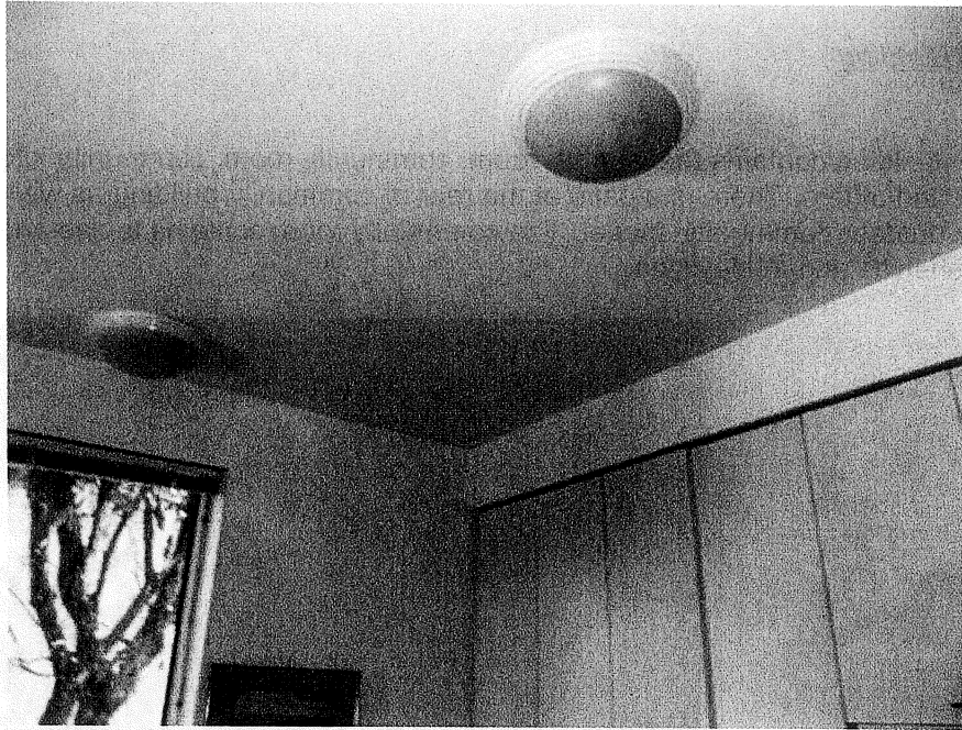
Typical ceiling fixtures at kitchen
