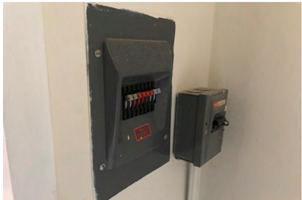
#42 UNIT ELECTRICAL PANEL
