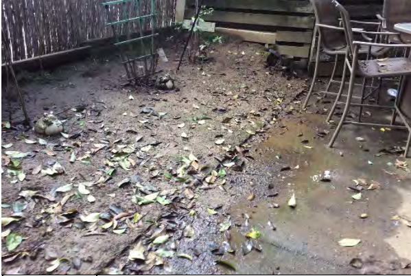
#43 PONDING WATER AT APT 3 PATIO
