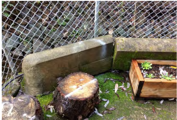
#46 BLOCK FENCE/BARRIER DAMAGE FACING CREEK
