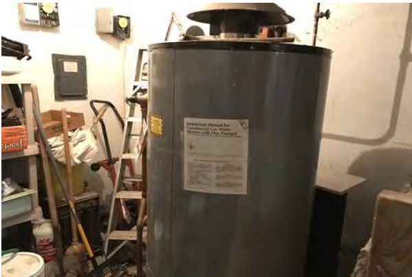
#23 DOMESTIC WATER HEATER
