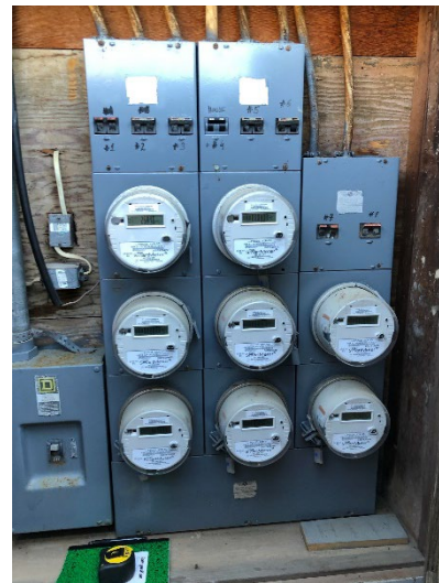
200 amp main breaker insufficient for 8 apartments
