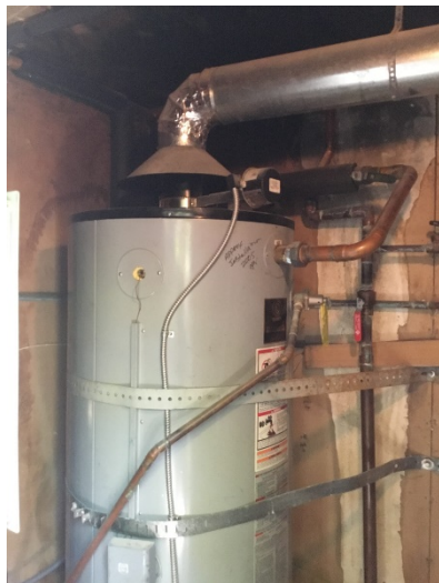
Ocean Terrace water heater showing soot on ceiling due to poor venting
