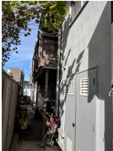
Ocean Terrace Apts, view of utility closet where water heater is housed
