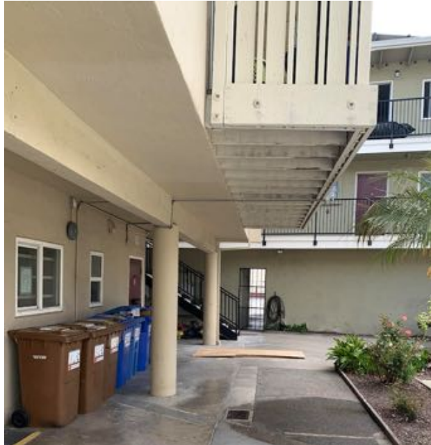
Ground floor near laundry – column supports and beam run under upper units. Cantilevered decks
