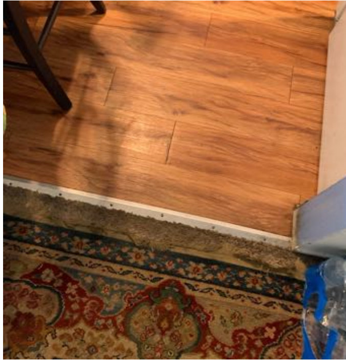
Sheet vinyl floor at kitchen, cut pile carpet at living room (covered by resident's rug)
