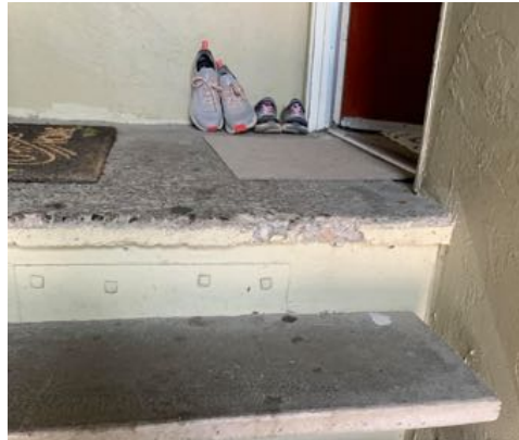
Stair landing – worn concrete topping
