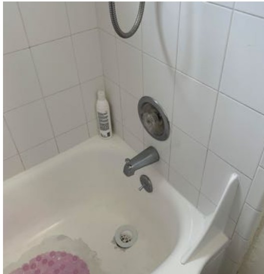
Shower surround and tub (peeling coating) at Unit 19
