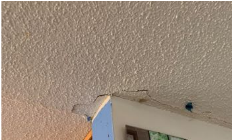
Settling at ceiling near kitchen at Unit 8
