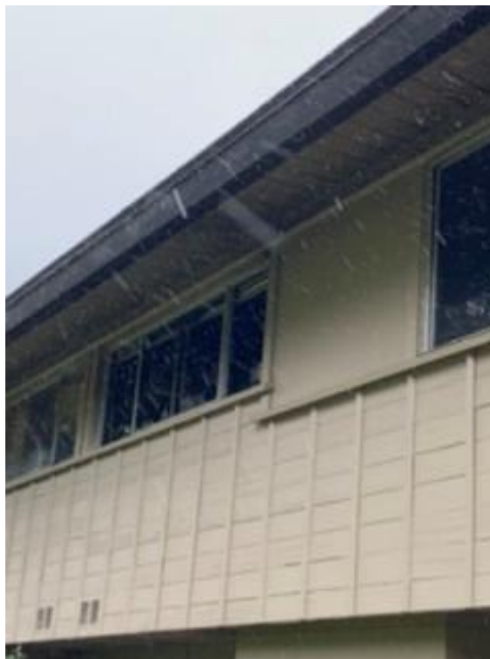
Figure 10: Photograph of low-rise building B-12 showing the exterior of unit 115 at the rear façade, facing southwest, with smoke damage at the windows and eaves. Source: MHA, received by ICF on 5/19/2020.
