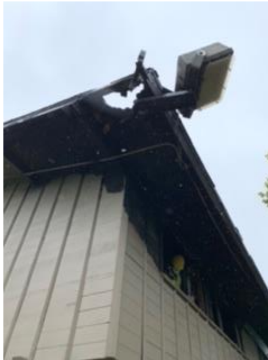
Figure 11: Photograph of building B-12 showing the exterior of unit 115, roof and siding damage at the primary (west) and north façades, facing southeast. Source: MHA, received by ICF on 5/19/2020.
