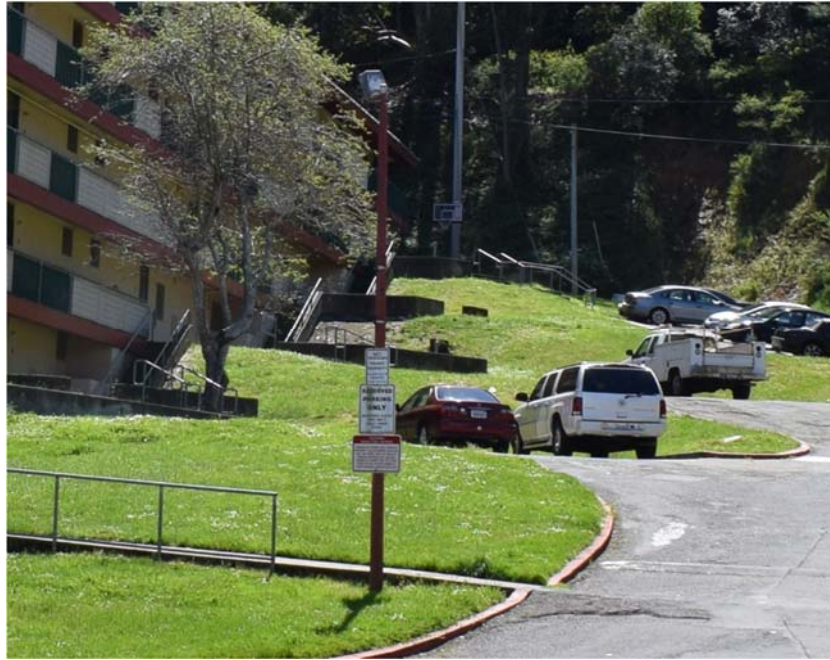
Figure 5. Representative example of the 20-foot Specific Area lighting standard in the parking area near the high-rise building at 89 Cole Drive, facing south. Source: ICF, April 2019.
