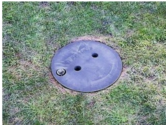
Photo 7 Example of an in-ground junction box. Source: MHA, 2023.
