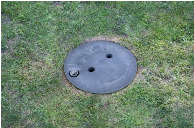
This is an example of an in-ground junction
