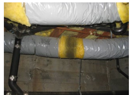
Leaky Duct Seam
