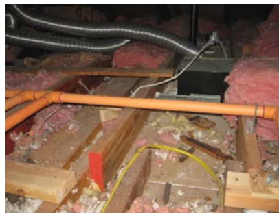
Poorly Insulated Attic
